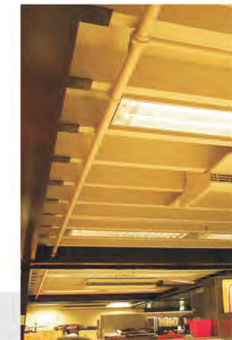
Utilized low height exposed unit to fit within 8.5" available space of a heritage building
